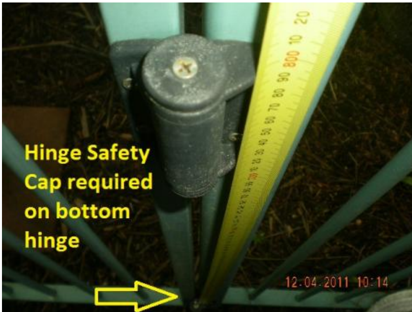
4. Safety hinge cap required.
