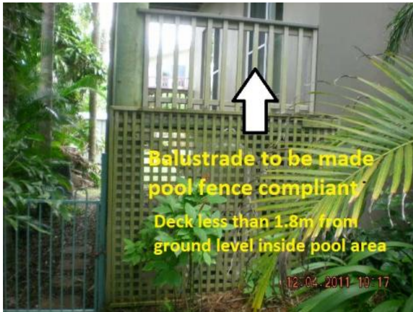
1. Balustrade to comply with QDC MP3.4 (Pool Fence compliant) Fig.22 as attached compiles with the part
